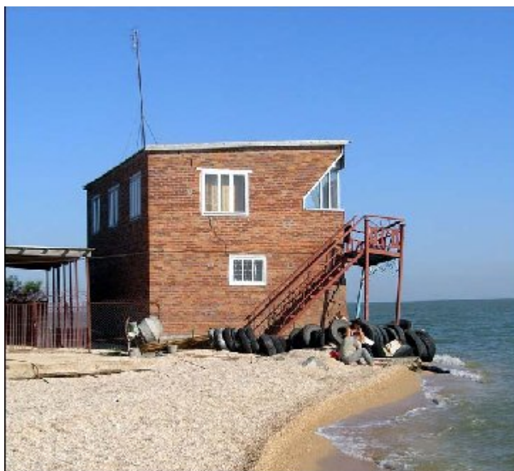
Partially damaged due to the coast washing out building located on the edge Figure 10: Partially damaged due to the coast washing out building located on the edge
