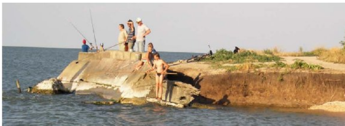
Figure 11: Eroded sea wall near sanatorium "Azov"
