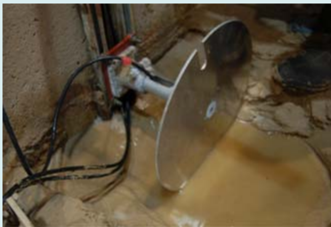
Installed as pressure sensor
